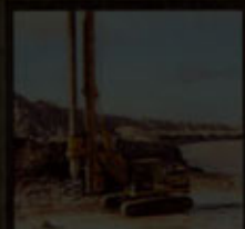
Stormwater Treatment Area 2 Comprehensive Engineering Restoration Project
